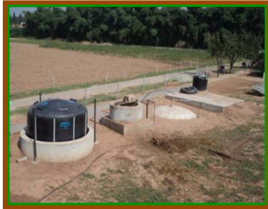
Fixed Dome and Floating Type Biogas Digesters
