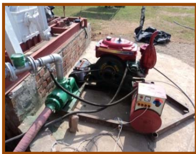
Dual Fuel Engine ( Biogas : Diesel \approx 62:38)
